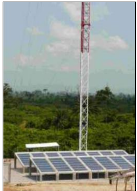
Figure 2: Solar powered BTS – Côte d'Ivoire
