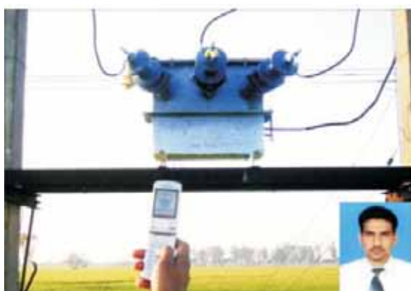
Electric transformer protection device
