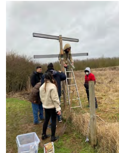
Fig. 13. Installation of a SmartSense Monitoring System by students, Germany
