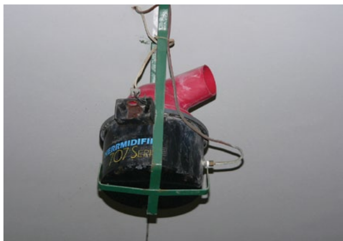
A storage room humidification unit
